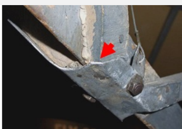
Fig. 1: Photograph of the aeroplane showing the location of the fixation plate (red dot) ( www.hepta.aero ),
