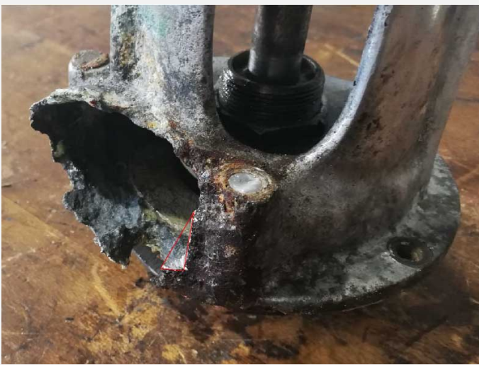
Fig. 5: Close-up view of the corroded exit pipe of the disassembled Hispano water pump, showing the sampled area,
